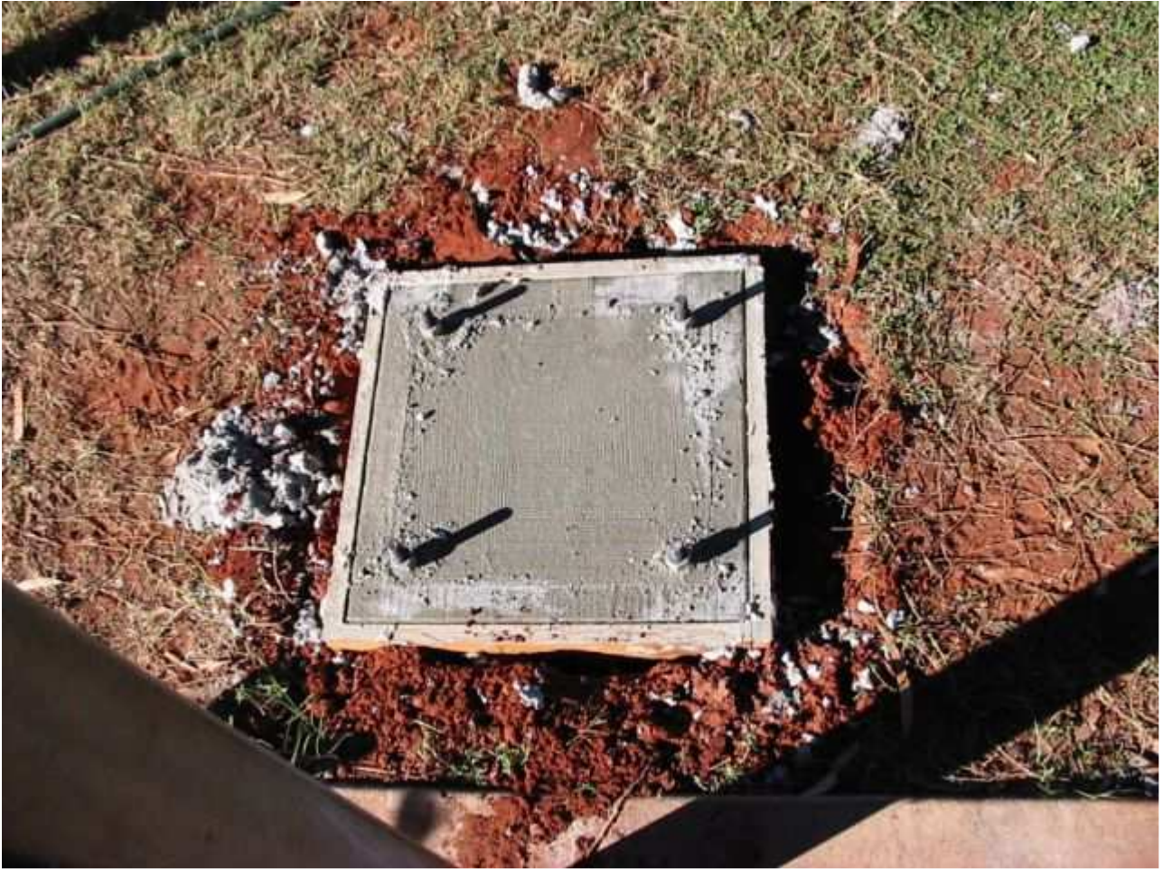
THE CONCRETE PAD. ABOUT 350mm SHOWN, BUT IT'S 500mm X 500mm SQUARE AND 850mm DEEP.
